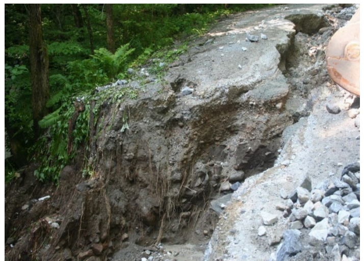
Major scouring on Sugar Hill Road in July 2023 (DR4720)
