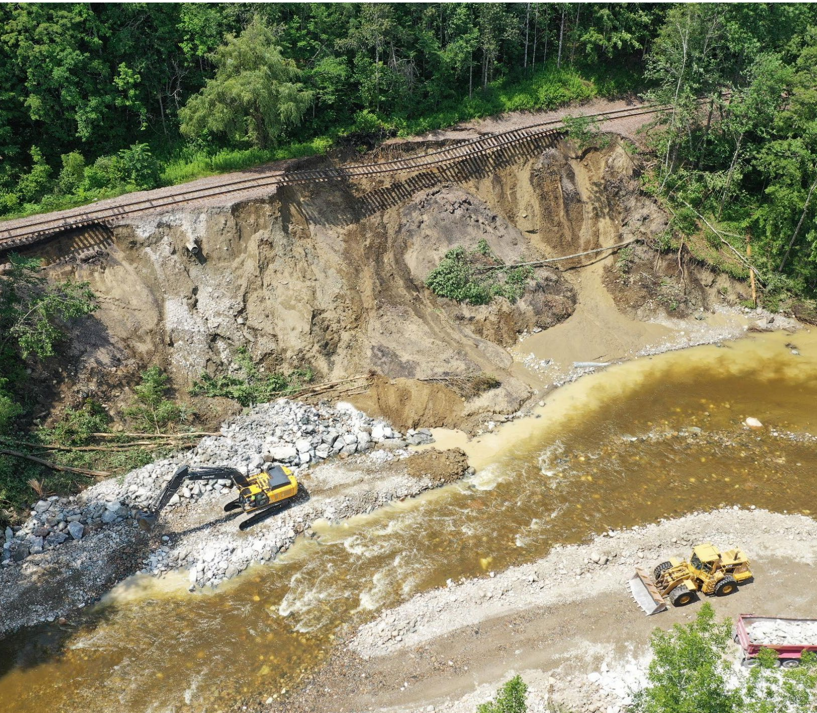
Fluvial erosion causing a slope collapse in East Wallingford, destabilizing a portion of the railway next to the Mill River (DR4720)
