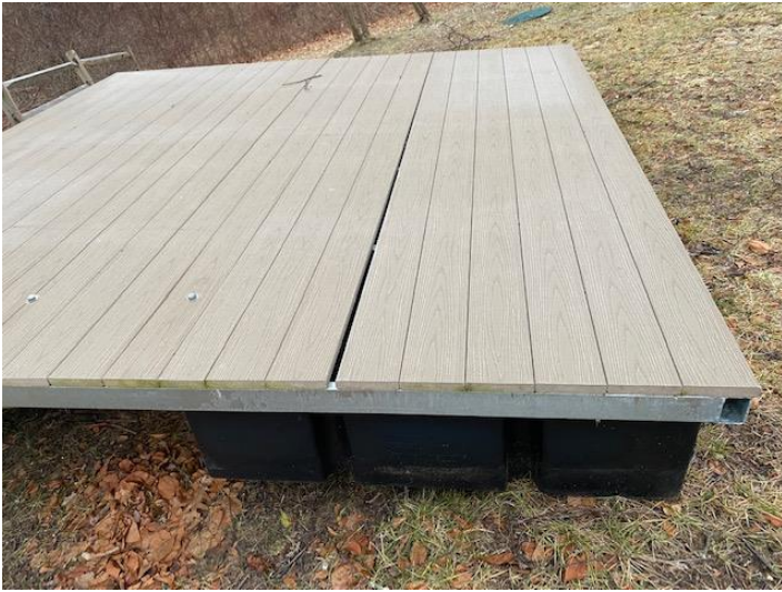
Pictures of deck separation on float:
