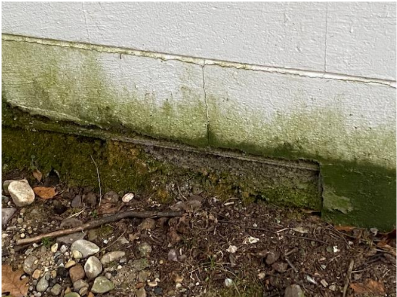
Pictures of North and South wall block erosion:
